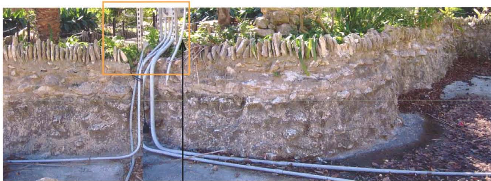
34 CAP MISSING BECAUSE OF EXTENSIVE PIPING IN AREA. REMOVE/PROTECT METAL CONDUIT/PIPE. HIDE WITH PROPOSED PLANTING. PAINT CONDUIT BLACK TO BLEND WITH LINER.
