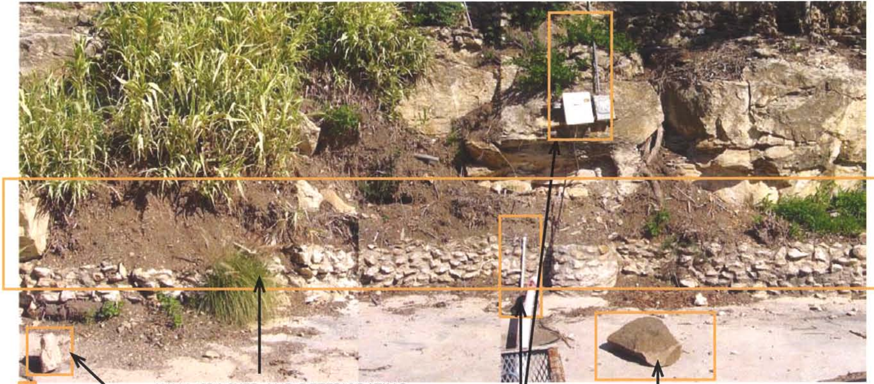
25 FALLEN ROCK WALL CRACKED AND DETERIORATING OR NOT EXISTING IN THIS AREA. INVASIVE AND OVERGROWN CANE TO BE REMOVED.
