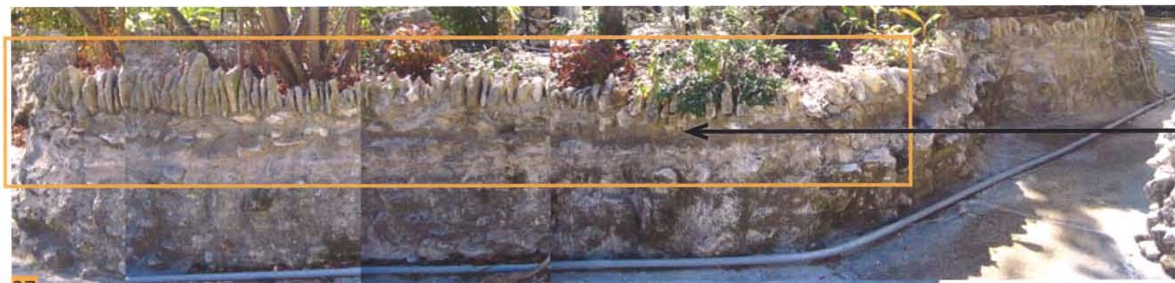
37 EVIDENCE OF PREVIOUS STONE CAP REPAIR.
