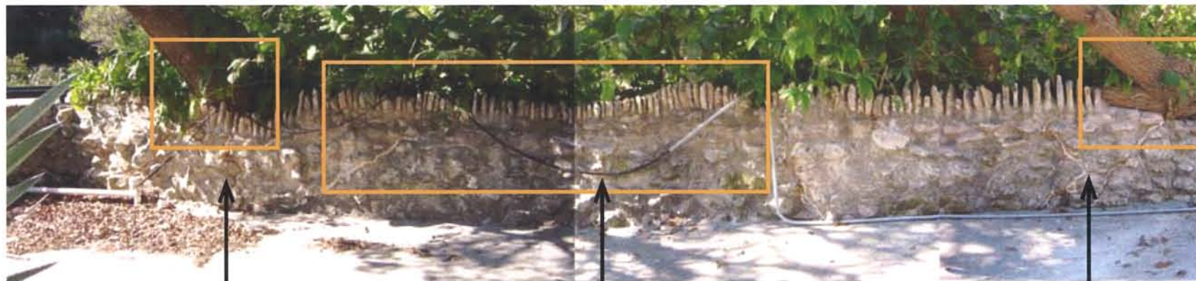
32 TREE ENCROACHING ON WALL. REMOVE CONDUIT. TREE ENCROACHING ON WALL. WALL REPAIRED IN PAST (SEE CRACK WITH MORTAR).
