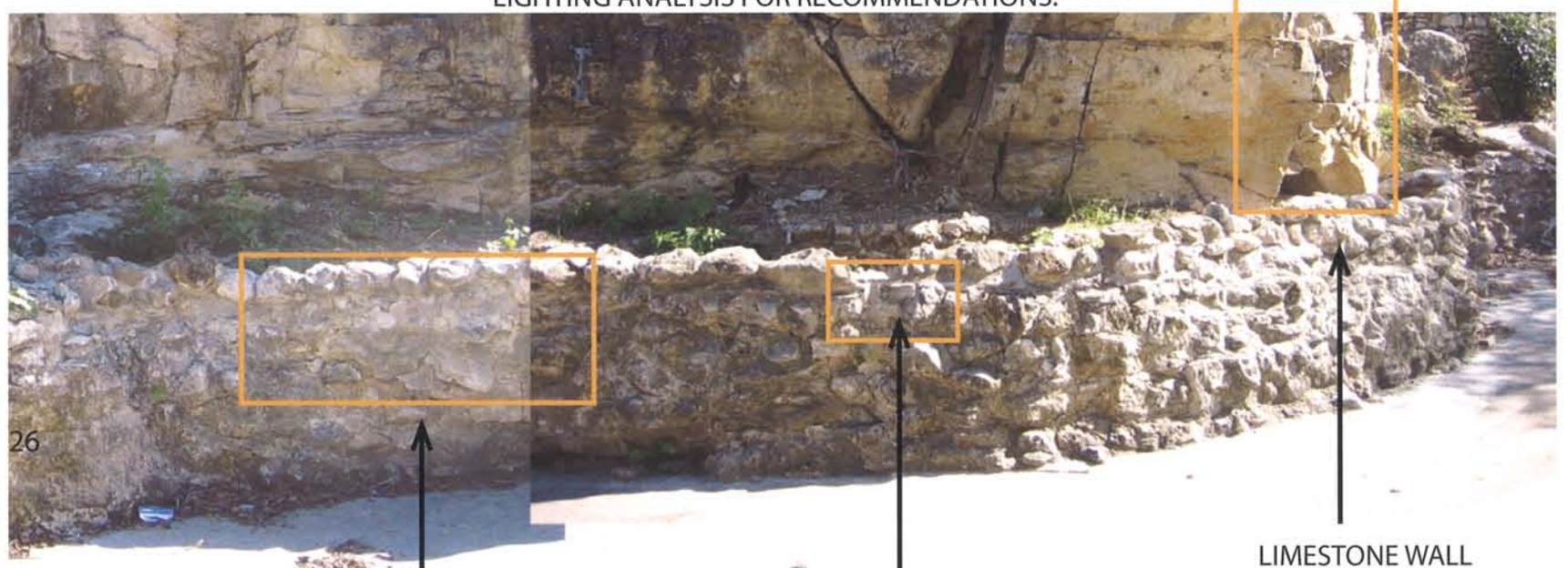
29 WALL CRACKED. STONE CAP MISSING OR DETERIORATING. LIMESTONE WALL DETERIORATING.
