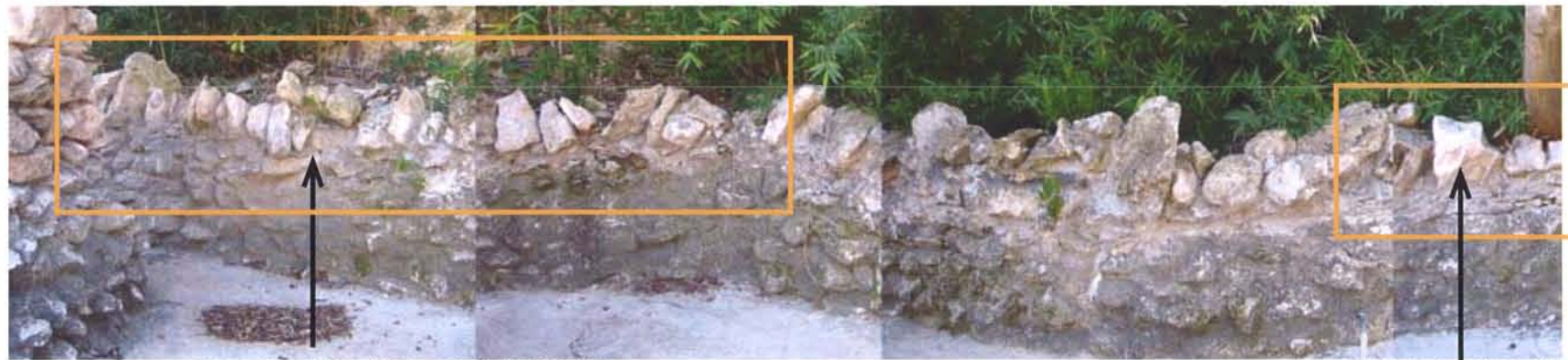
7 CAP CRACKED AND DETERIORATING OR MISSING.
