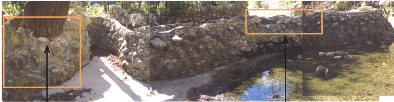
17 TREE PUSHING OUT AND COMPROMISING WALL.
