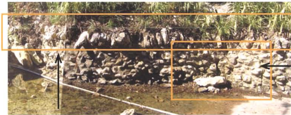
18 INVASIVE AND OVERGROWN CANE COMPROMISING STONE CAP. WALL IMPACTED BY ROCK SLIDES.
