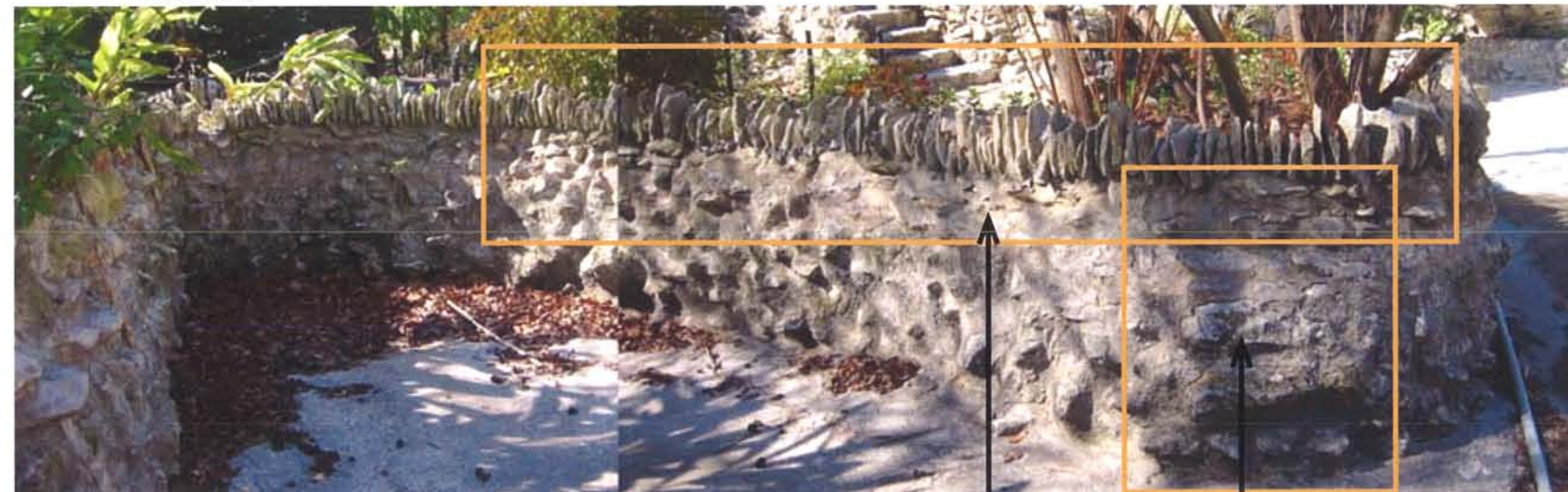
36 EVIDENCE OF PREVIOUS STONE CAP REPAIR.
