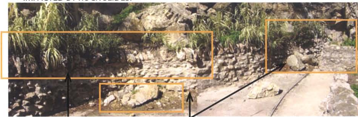
19 STONE CAP COMPROMISED
