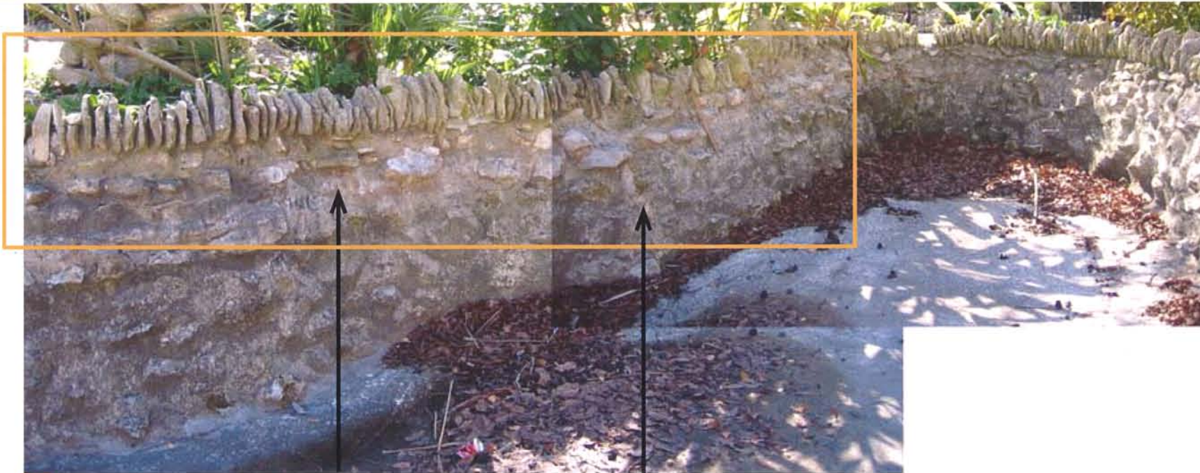
35 TOP TWO FEET OF WALL CRACKING AND DETERIORATING. EVIDENCE OF PREVIOUS REPAIRS.
