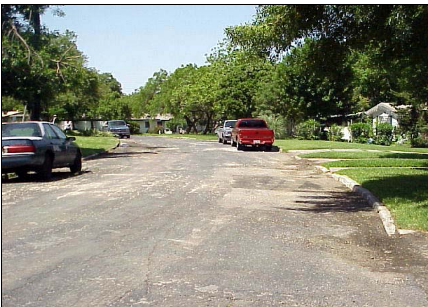
Example of a street in bad condition, Francis Jean Street.
