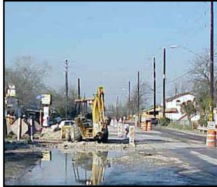
Far left: New sidewalk construction by Japhet Elementary School. Left: Reconstruction of Clark Avenue.
