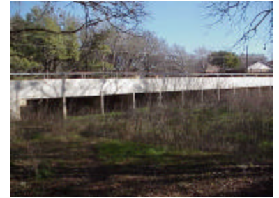
The Whitby Road Bridge over Huebner Creek replaced a neighborhood low water crossing.
