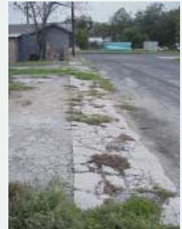
An example of a sidewalk in need of reconstruction within the neighborhood
