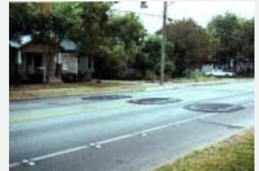
Speed cushions are positioned to fit the wheel base on fire trucks.
