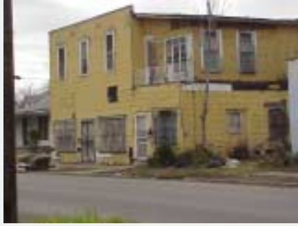
Example code compliance problem in the neighborhood
