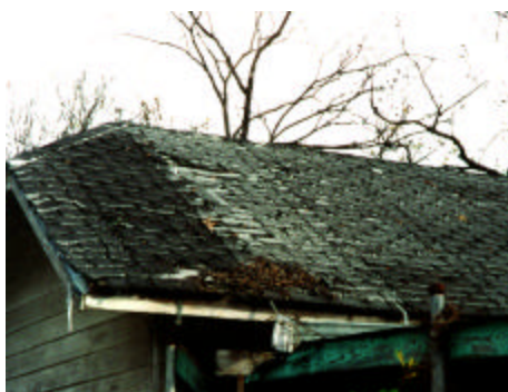
Examples of houses in poor condition with potential code violations
