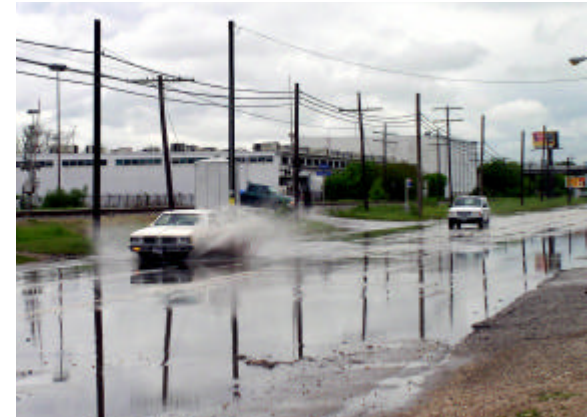
Frio City Road drainage problem.
