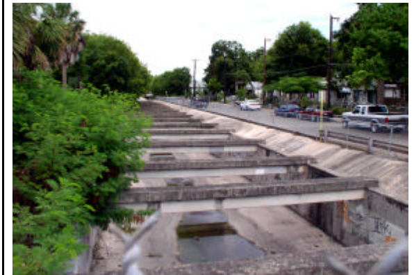
Concepcion drainage channel at Nogalitos
