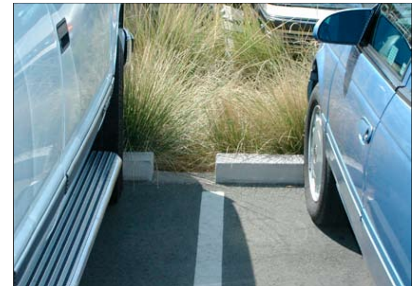
Left: Depressed parking lot islands provide area for water runoff and decrease the need for storm sewers.
