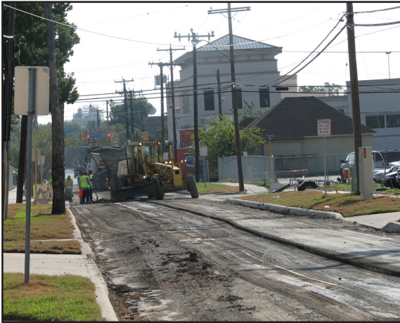
Street construction, such as this on Dewey and McCullough, should be comprehensive thus improving the overall value of the neighborhood.
