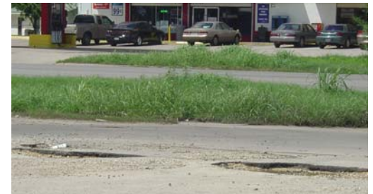
Pavement Repairs Needed along Old US HWY 90
