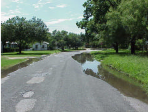
Neighborhood experiencing poor drainage during and after rain.
